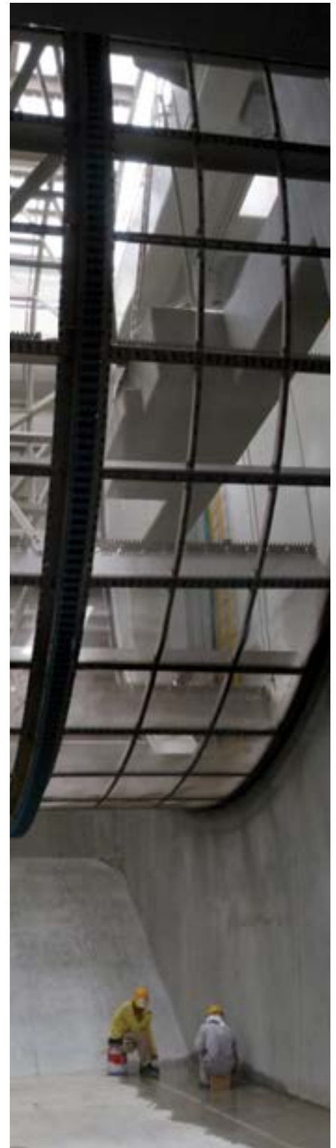
Underneath of a DE drum screen
