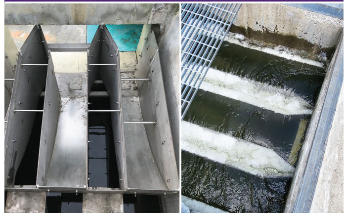
SERPENTINE WEIR CONTROLS
